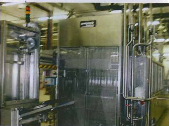
Packing material (here: cups) is transferred to the fillers from the basement
